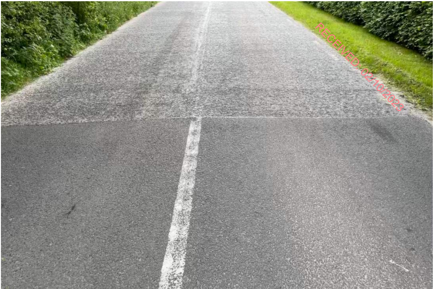
Picture B3: Section A - Chainage 165 – Transverse Joint between SMA and HRA surfaces
