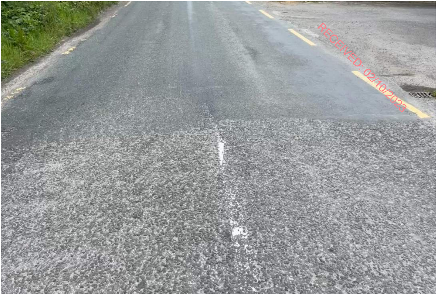
Picture B7: Section A – Chainage 890 - Transverse Joint from HRA to older surface
