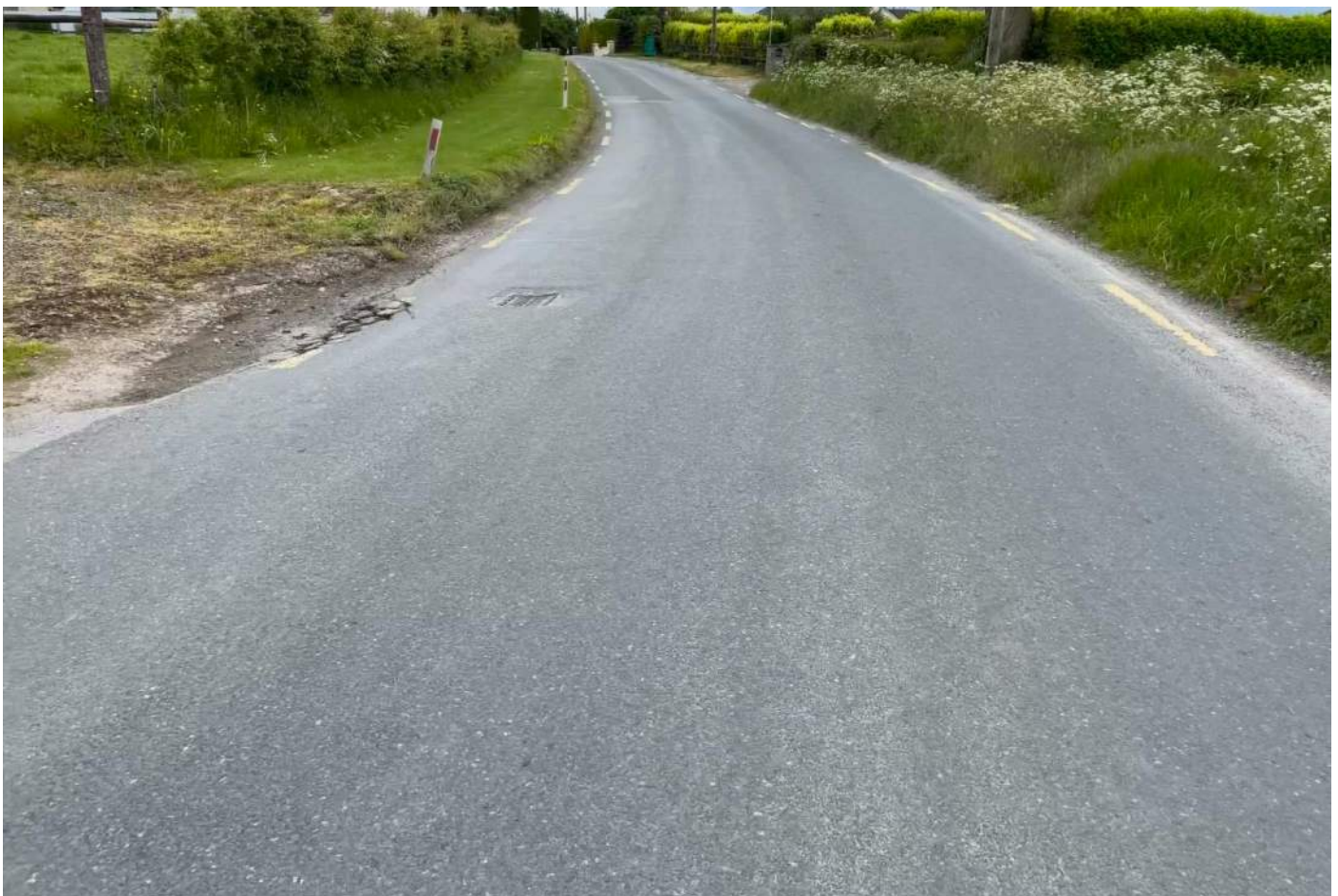
Picture B10: Section B – Chainage 2080 – Gully and Edge Damage
