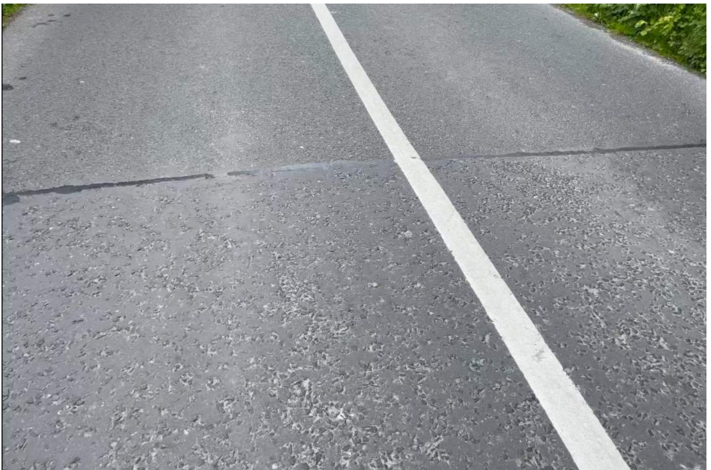
Picture B2: Section A – Chainage 45 – Transverse Joint between HRA and SMA surfaces
