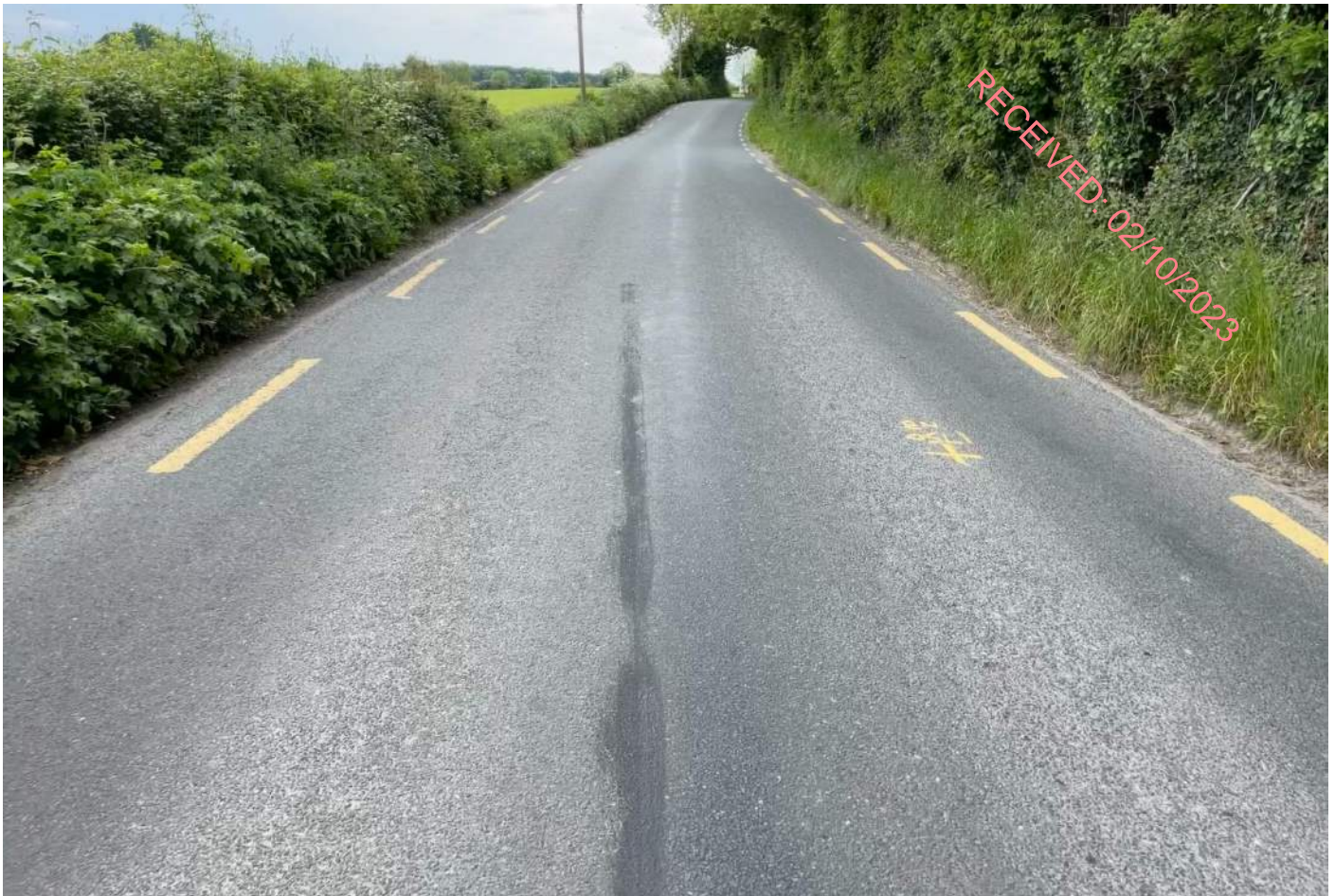
Picture B9: Section B – Chainage 1750 – Bleeding in wheel-tracks
