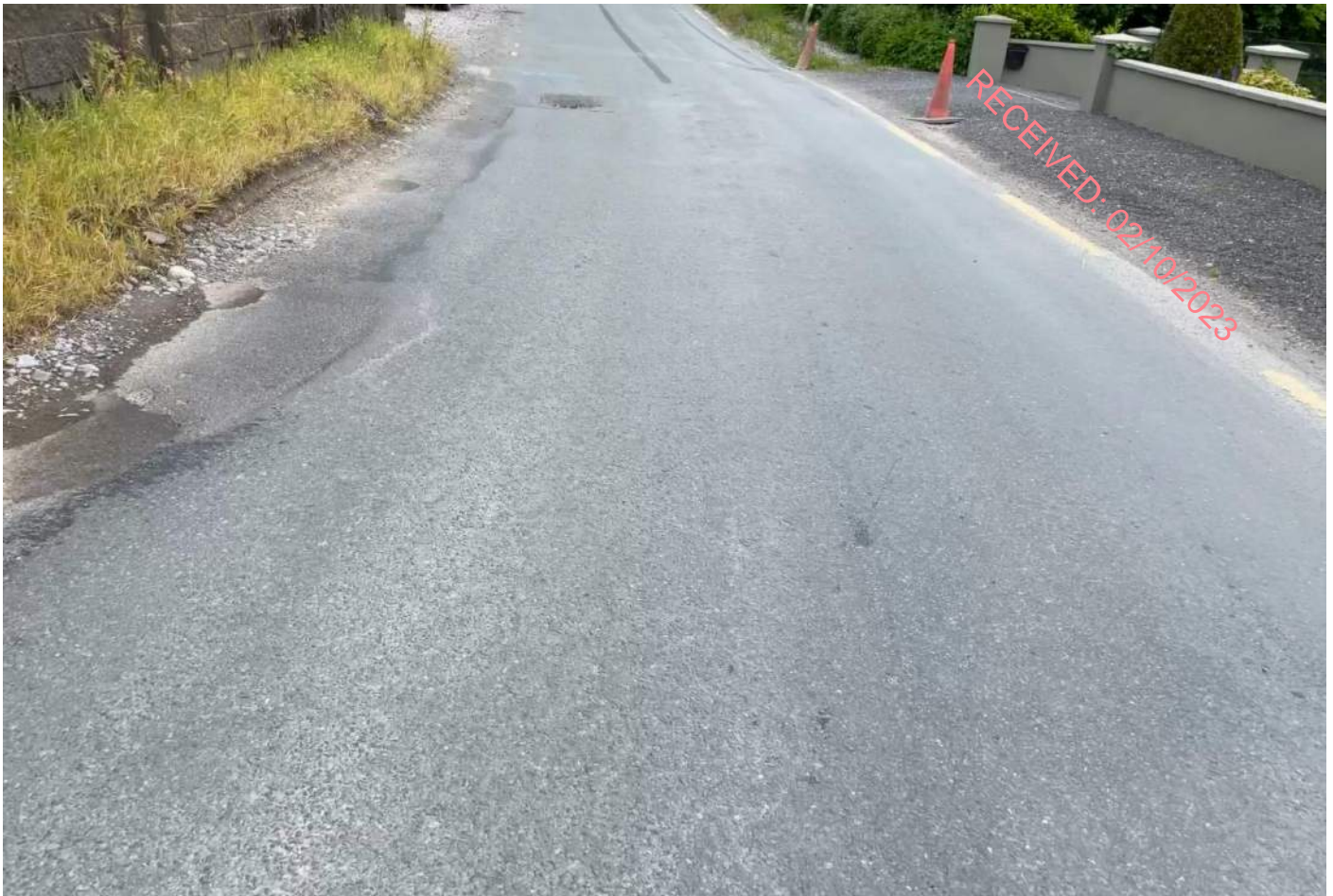
Picture B11: Section B – Chainage 2200 – Patching/Edge Damage
